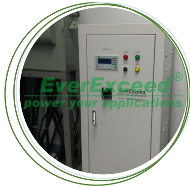
The Phillipines NGCP substation uXcel 125V200A charger
